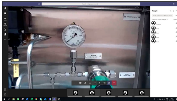
Typical remote commissioning session in execution
